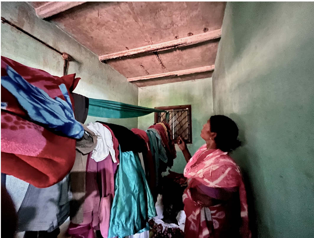
Choudamma inside her house at the resettlement colony. The roof and walls began to show signs of seepage during the second monsoon after their arrival, she said. Her family lives in a more traditional structure they
