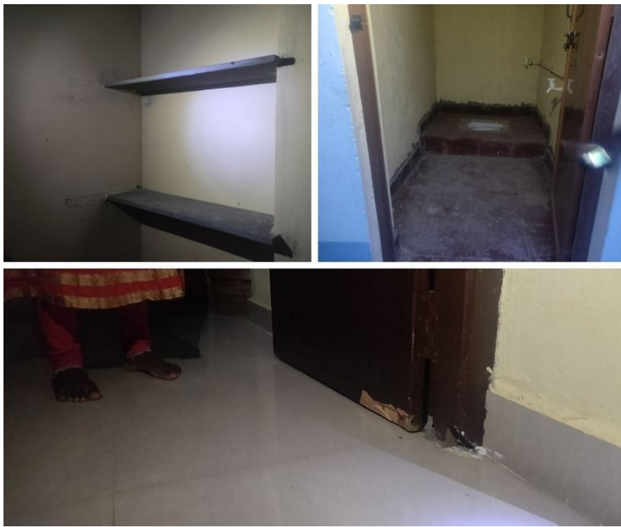
Cracks and leaks at the resettlement site. Greeshma Kuthar/Firstpost
